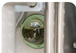
Oil sight glass with autostop
